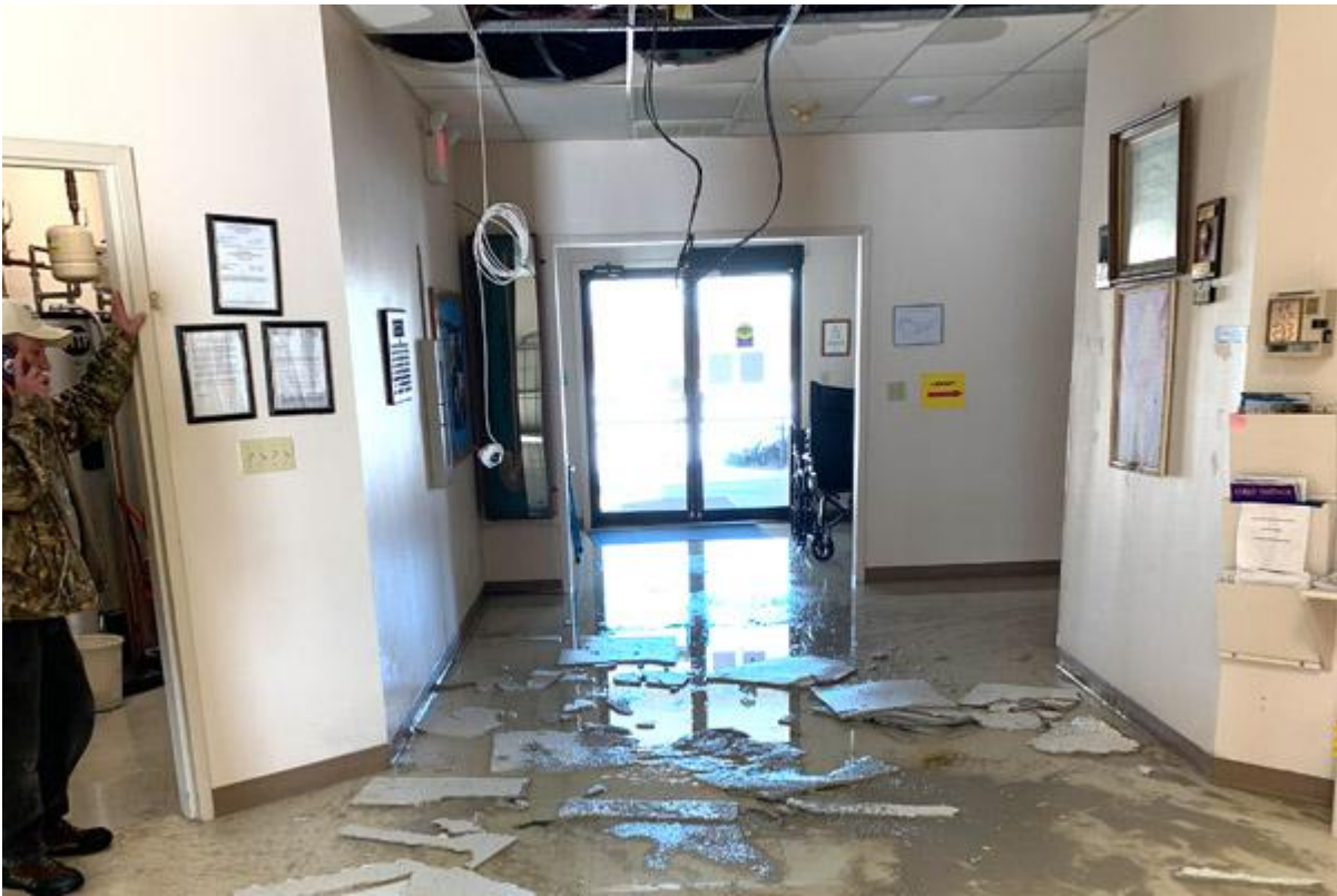
A frozen pipe in the ceiling of St. Bernard Church's parish hall soaked ceiling tiles in several areas and dumped water in the entrance way. Both the hall and church were damaged by burst frozen pipes during the night of Feb. 16. According to the metering system, 10,000 gallons were leaked within three hours. (Don Schmutz photo)
